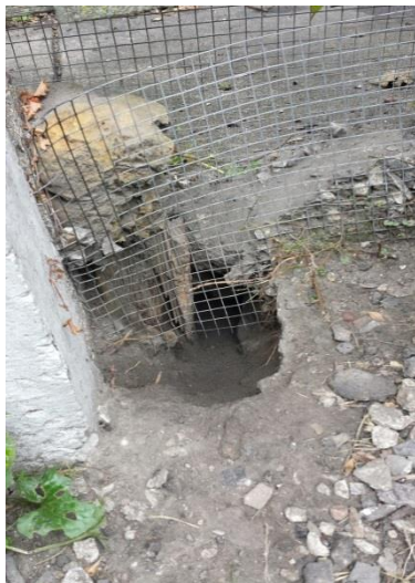
Fig. 2 Rat hole under fencing
